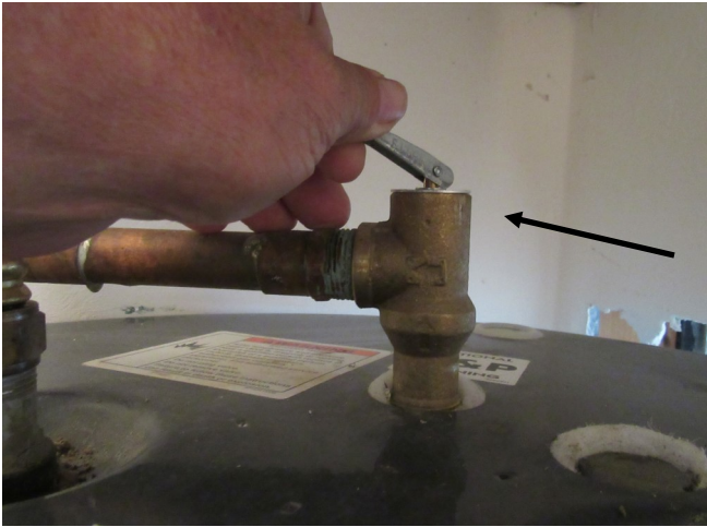
The pressure relief valve on the water heater did not release when tested.
