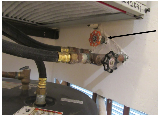
Water shutoff located above the water heater.
