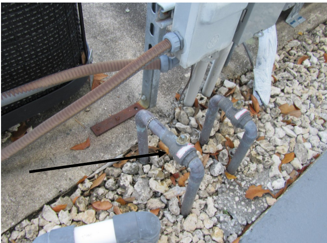
Water shutoff located by the air compressor
