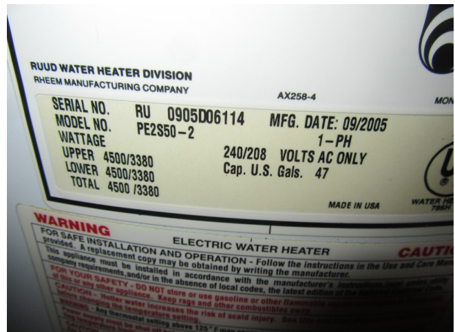
Water heater located in the 1st floor closet under the stairs
