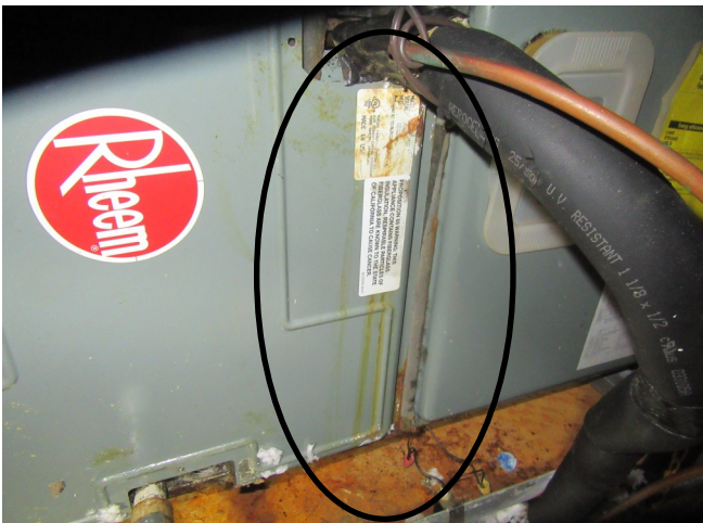
On the exterior of the air handler case, where the coolant piping connects to the coil, dry rust stains were noted running down the front of the case. There was also a noticeable quantity of dry rust in the bottom of the emergency backup overflow condensation pan under the unit.
