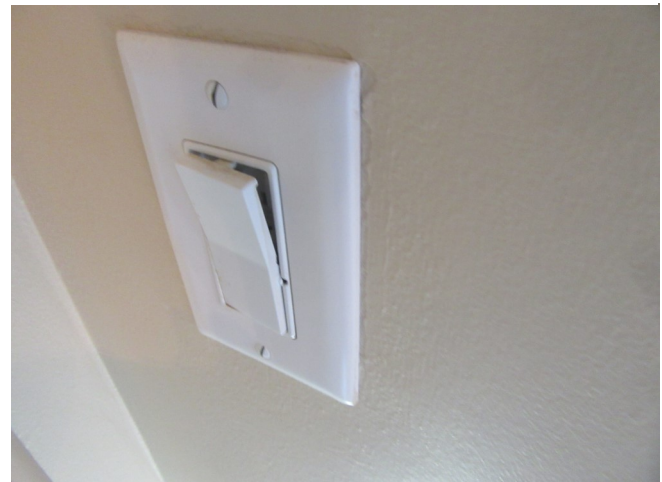
At a number of locations approximately 10 wall switches were noted to have their rockers (push buttons) coming loose..
