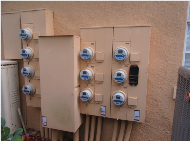
Electric meter and main breaker located in the south side of the building
