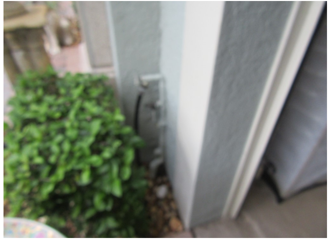
Main water shutoff located on the front of the building left of the garage door.
